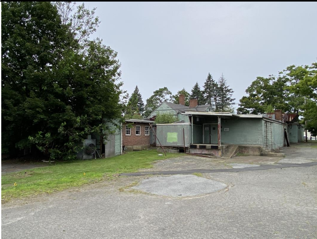
Southeast wing from SE. This flat-roofed, utilitarian structure of concrete block, ca. 1957-1961, housed the restaurant kitchen.
