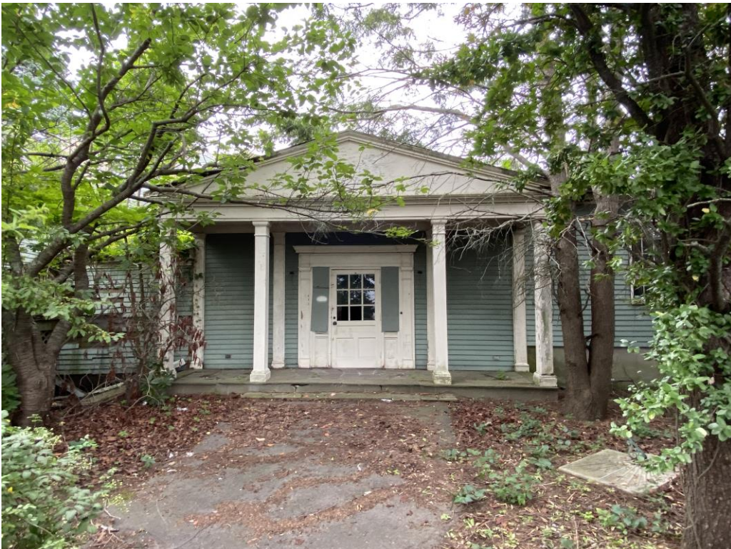
Main mid-20 th -century entrance centered on west-facing elevation, view from W.
