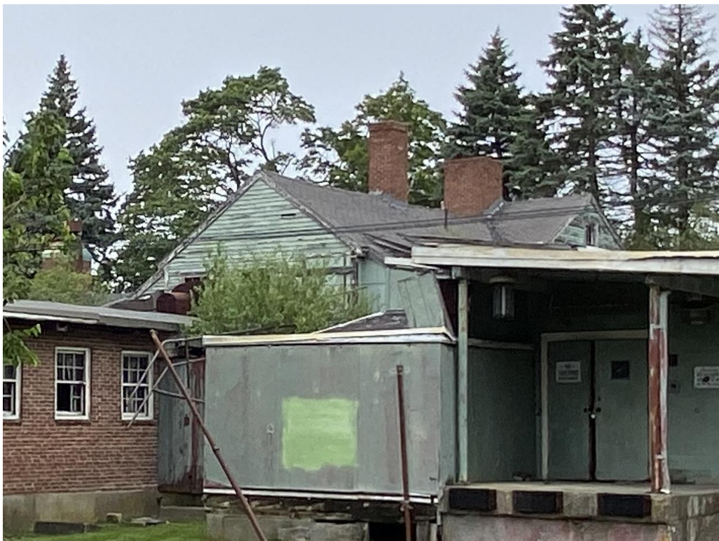
The same image, enlarged, showing the two-story 18 th century core of the building from the south.
